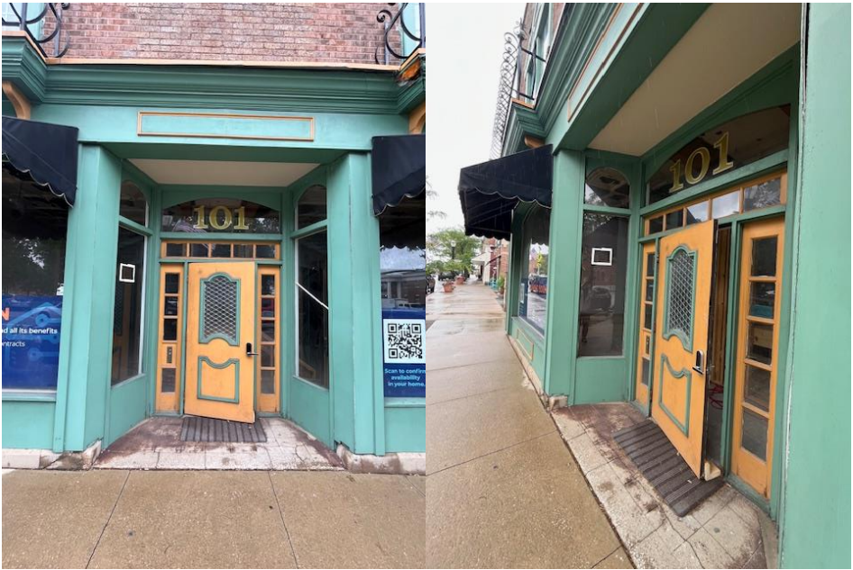
Exterior door and remaining lites to remain, to paint, like colors.
